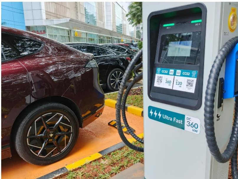
Figure 11. Typical high-power DC fast-charging station equipped with a CCS connector. Source: Adapted from Energy Reports [5].
